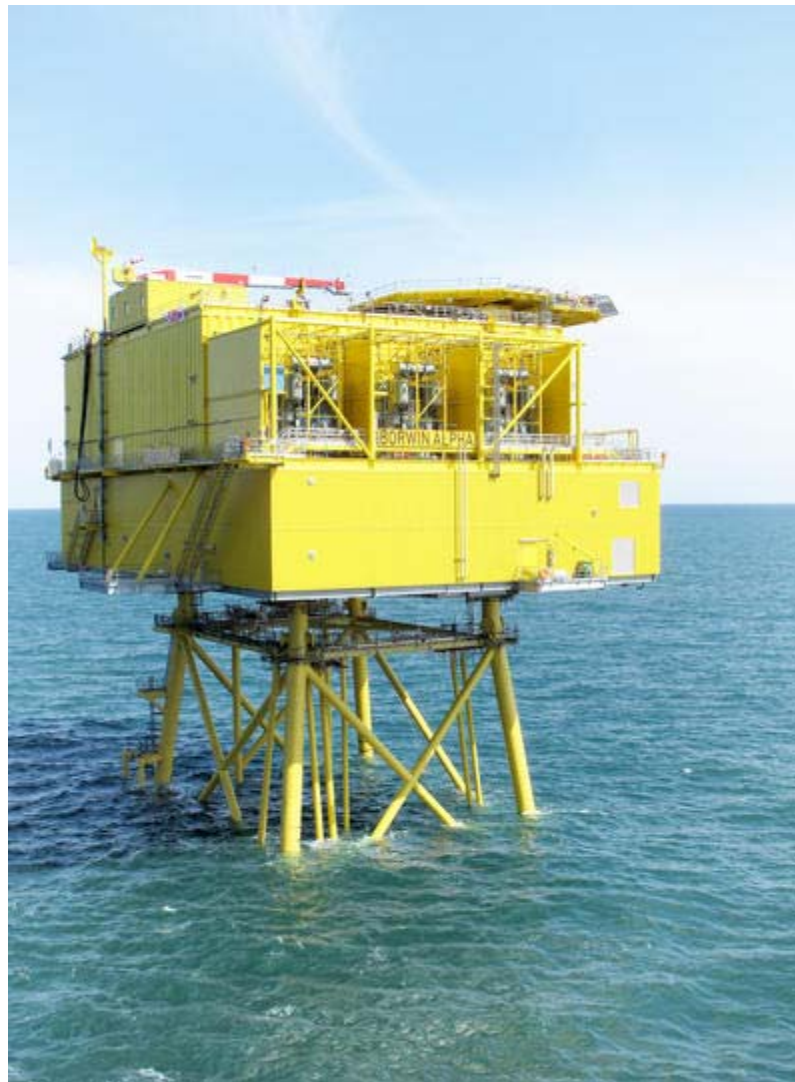
FIGURE 6. BORWIN ALPHA OFFSHORE CONVERTER STATION (COURTESY OF ABB)
