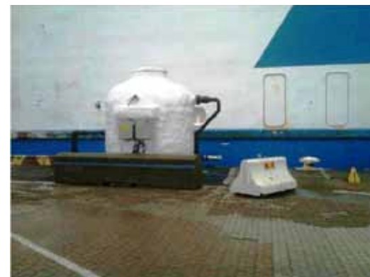
Port Reception Facility for ship sewage at the Port of Trelleborg.
